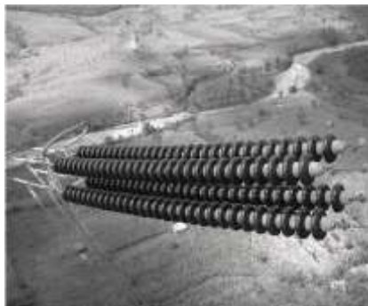
Gambar 2.27 Isolator Quadruple String
