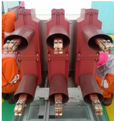
(a) CB/ PMT 20 kV Belakang
