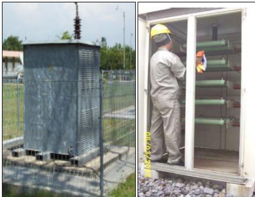
Gambar 2.11. Neutral Grounding Resistor (NGR)
