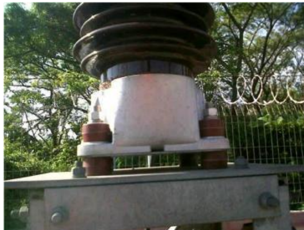
Gambar 2.15 Insulator Dudukan Lightning Arrester
